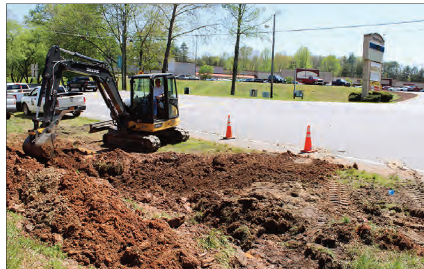
An employee with the Town of Franklin said the waterline break likely occurred due to old pipes. Photo by Vickie Carpenter
