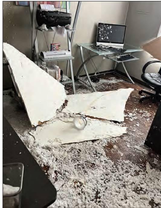
A severe temperature drop over the Christmas holiday caused extensive damage to the REACH of Macon County shelter due to a bursted pipe in the sprinkler system. The resulting flood sent the ceiling crashing into the shelter along with several inches of water. Photos submitted
