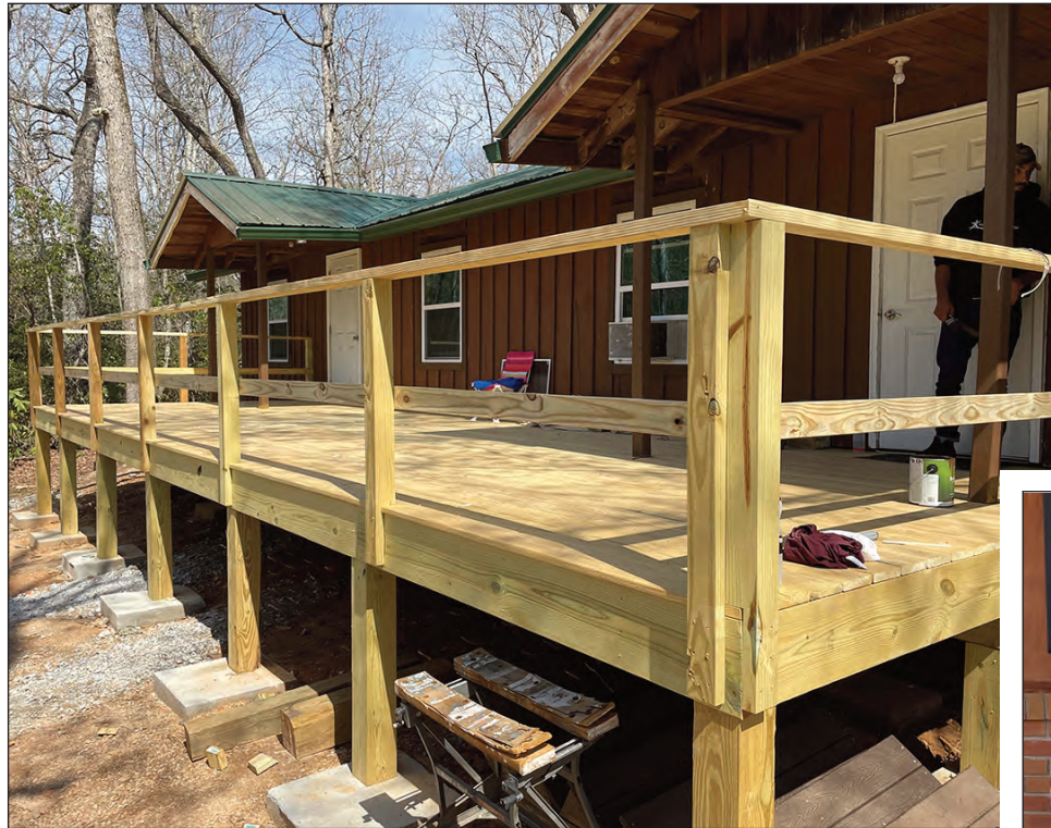
One of the many projects completed this year at the Men's Teen Challenge of the Smokies campus is a new deck on one of the housing duplexes.
