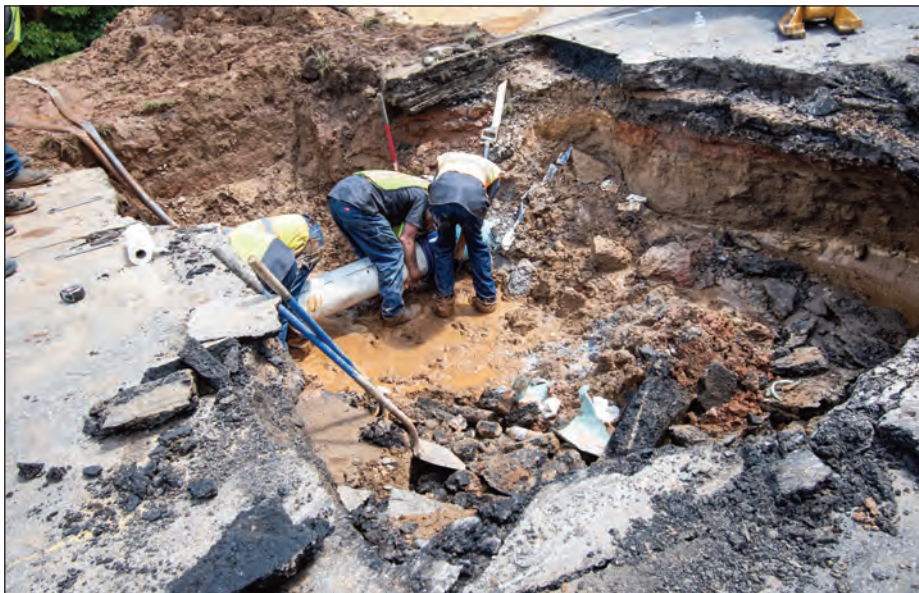
The water line break on Porter Street resulted in downtown businesses being without water for a short period of time on Friday afternoon. Town employees repaired the break but not before 200,000 gallons of water were lost.
