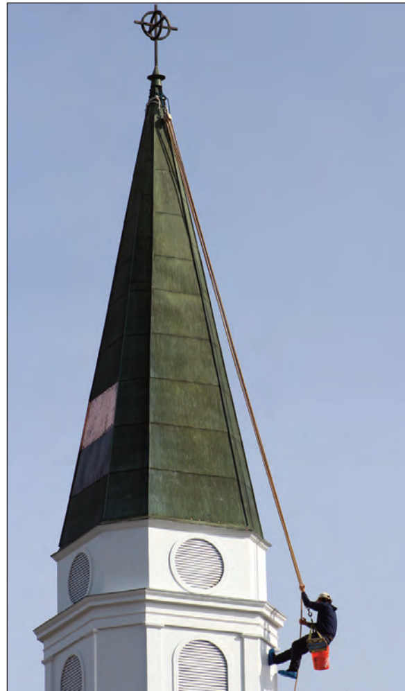
Repairs were recently done on the First Baptist Church steeple in preparation for the churches 200th anniversary. photo by Vickie Carpenter
