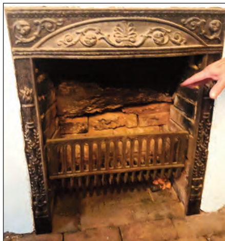
Most of the architectural elements were retained and restored including the grates on the fireplaces and the brass fixtures on the doors.
