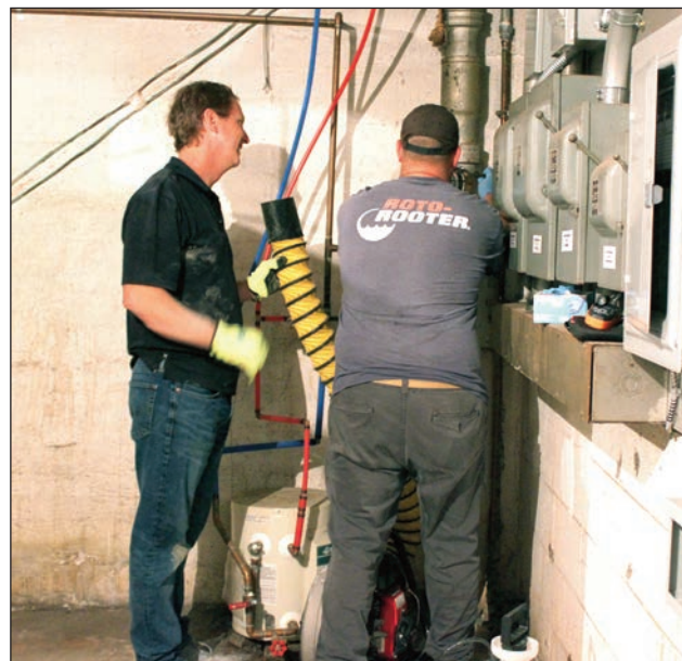
Roto Rooter Plumbers of Valdosta, Ga., did a smoke test on drain pipes and sewer lines of the building that houses Rust & Relics revealing leaks on all three levels.
