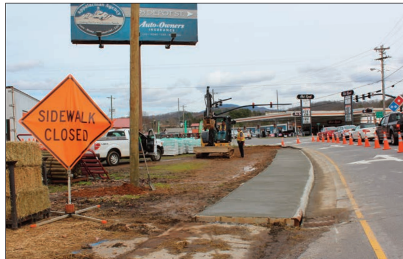
Town workers finish up a sidewalk project on East Main Street. The Town Council has made revamping sidewalks a priority. Photo by Vickie Carpenter
