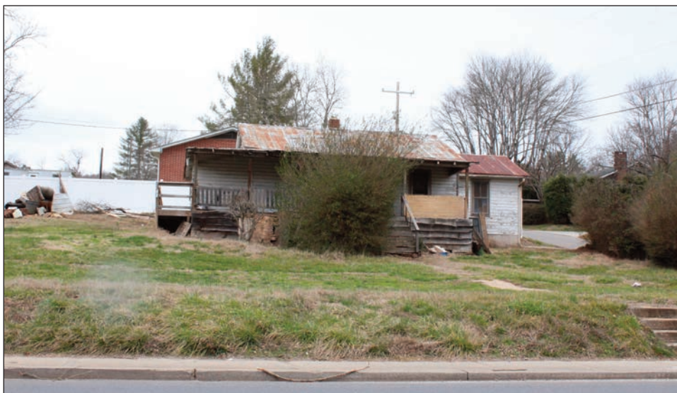
This vacant property on Wilkie Street is under consideration by the Town of Franklin to be cited under the Minimum Housing Ordinance. A hearing will determine the next course of action and whether or not the owner plans to clean up the property or face demolition.
