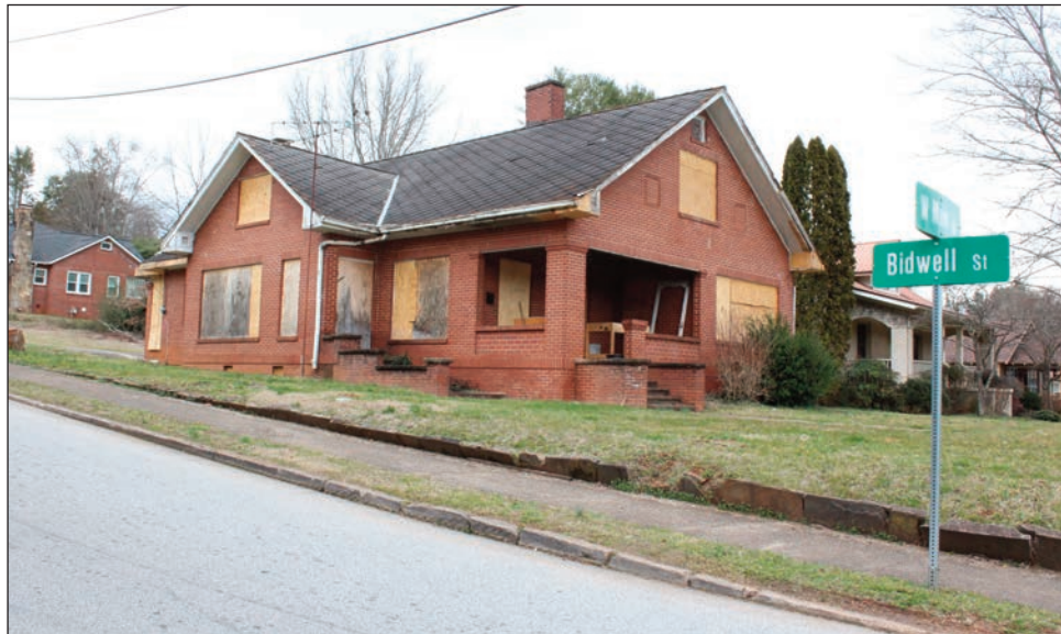
The owner of this Bidwell Street property has met the minimum housing code standard of making it “weathertight and watertight.” The town has dropped its lawsuit against the property owner.
