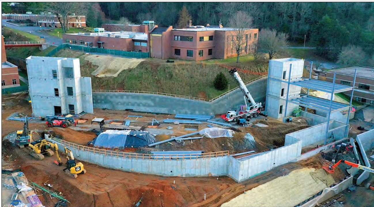
This aerial photo, taken on Jan. 1, shows the construction site of SCC's new Health Sciences Building in Sylva.
