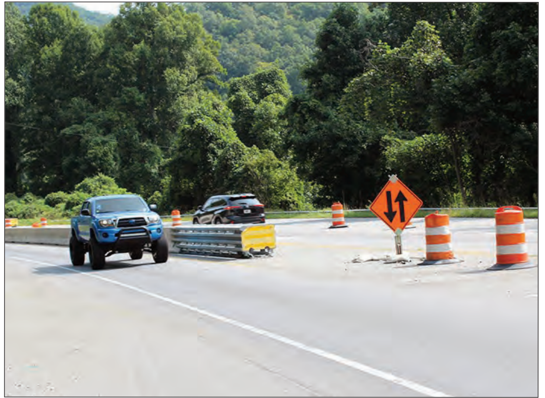
State officials are confident that the $6 million in repairs to the road on Cowee Mountain will last well into the future. The project is slated to be completed Aug. 1, 2021. Photo by Vickie Carpenter
