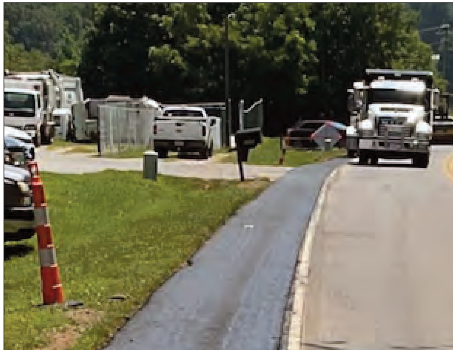
Improvements to the shoulders and the addition of reflective rumble strips on U.S. 64/N.C. 28 are designed to reduce crashes.
