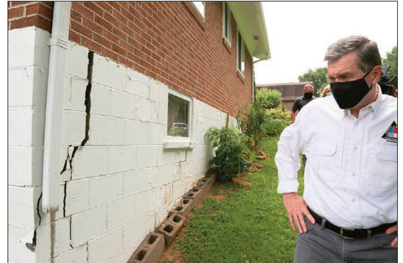
Governor Cooper visited Sparta on Tuesday to survey the damage caused by Sunday's earthquake. Photo provided
