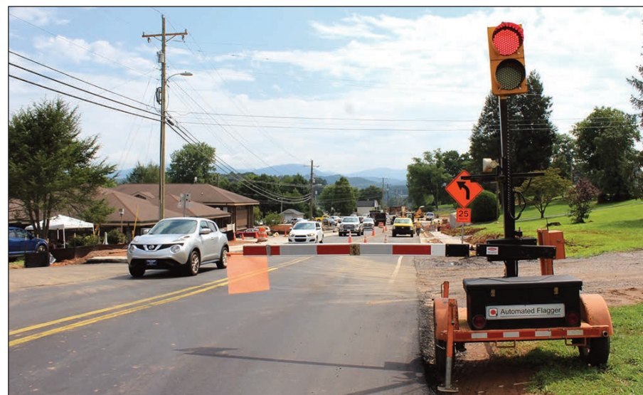
The final roundabout is under construction and is located within sight of the Maple Street roundabout. The sidewalks are also being reconstructed. Photos by Vickie Carpenter
