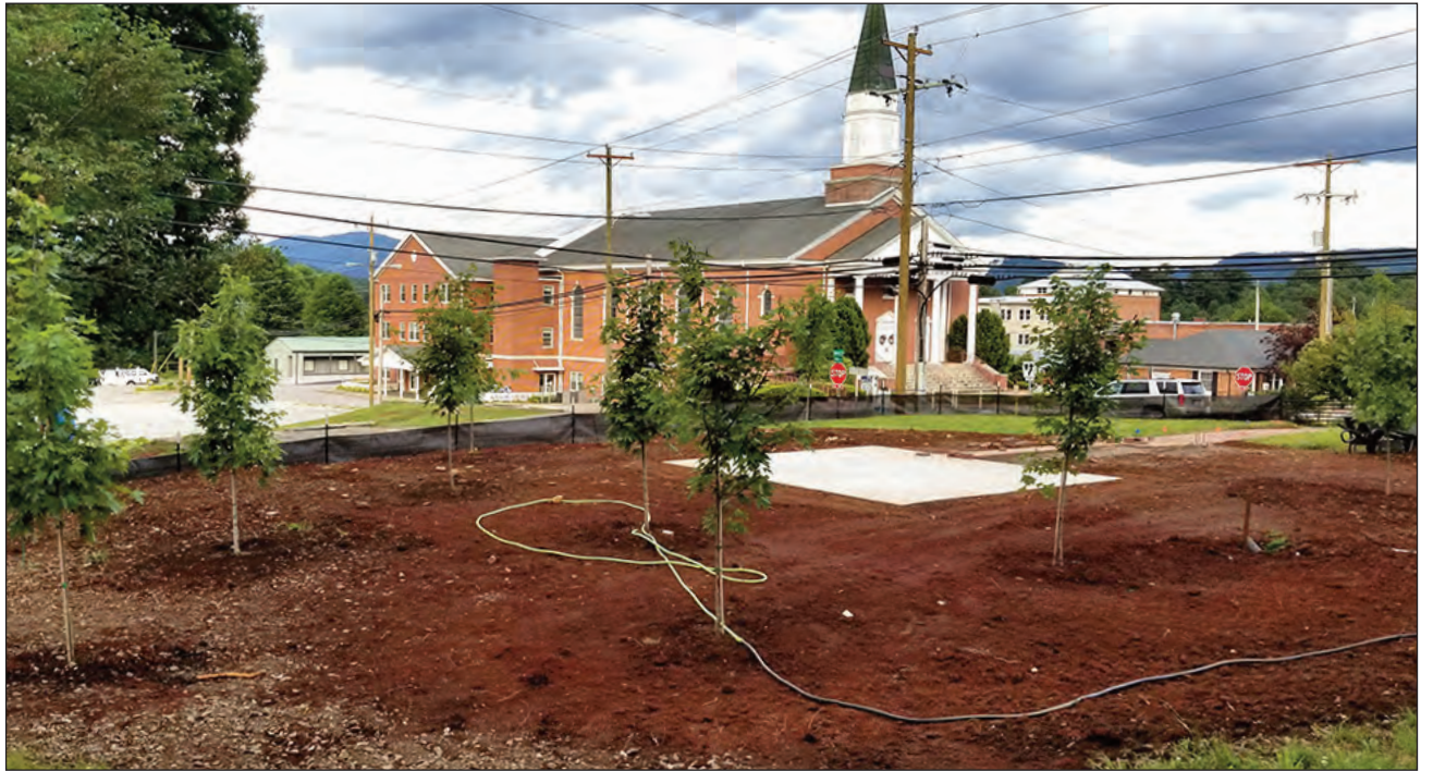
The Grove will consist of a timber frame pavilion, walkways, trees and other plantings to provide a quiet place for prayer and reflection.
