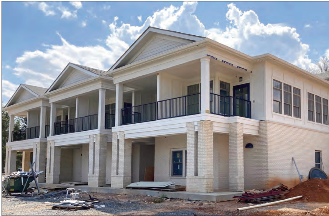
The new Hospice House currently under construction is located on Maple Street in downtown Franklin.
