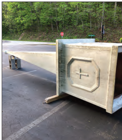
Removing the steeple from Cartoogechaye Baptist Church to clean and repaint it required a crane.
