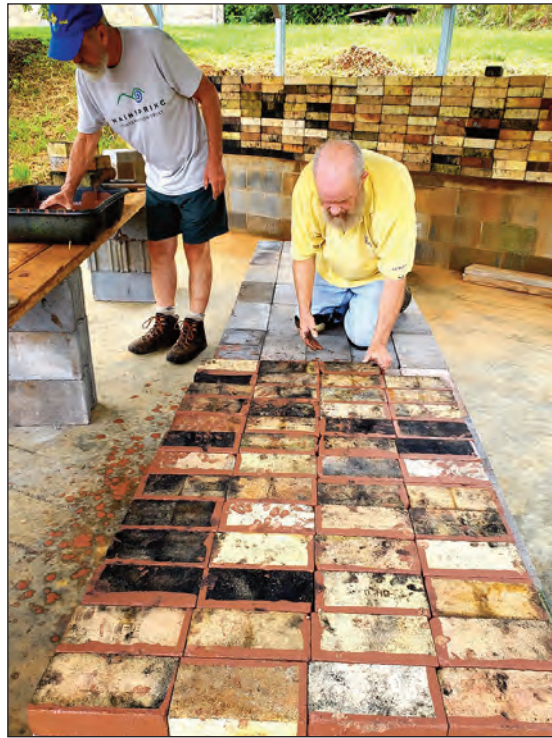
Construction of the wood-fire kiln began last fall and requires both porous and dense bricks, however the kiln has been in the planning stages for about three years.
