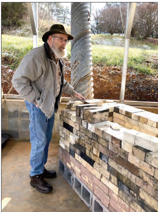
Potter Doug Hubbs explained the construction project and the reasons why a wood-fire kiln is an authentic and traditional method of firing clay pots. Photos by Deena C. Bouknight
